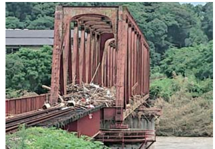
JR 肥薩線鉄橋損壊
